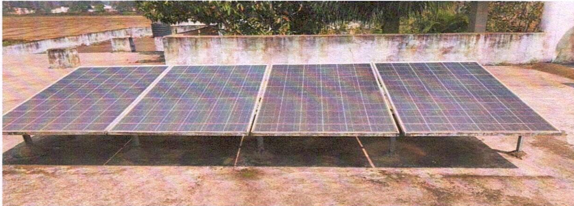
Solar panels arranged on the roof of Science block
